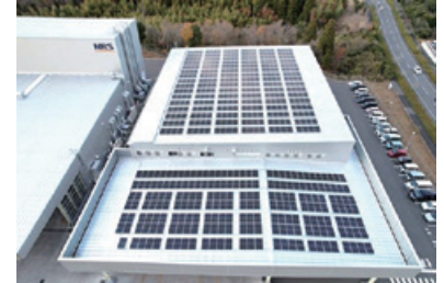
Solar panels installed at the Toke Distribution Center
